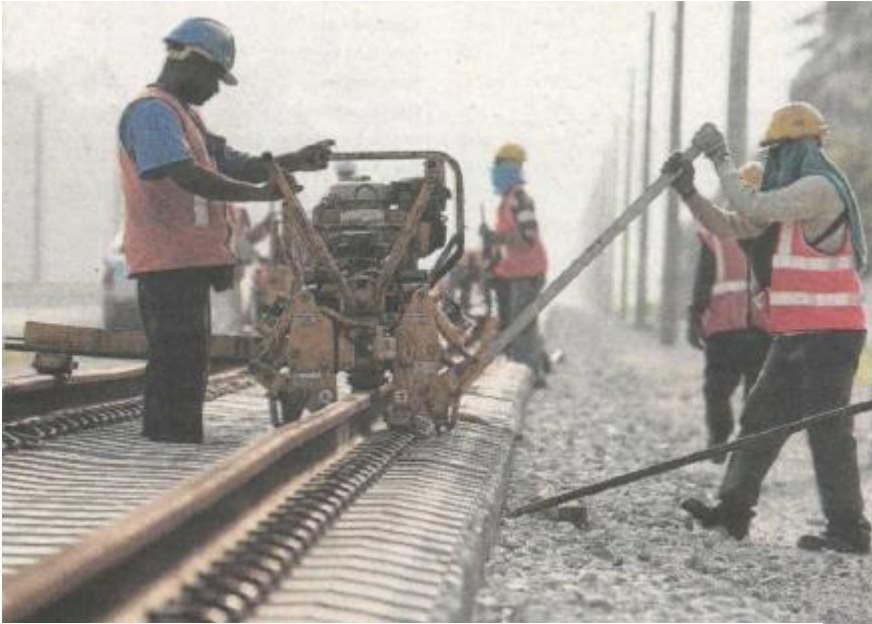
Workers conducting rail clipping works at the Bukit Gantang stretch of the Ipoh-Padang Besar rail track.
