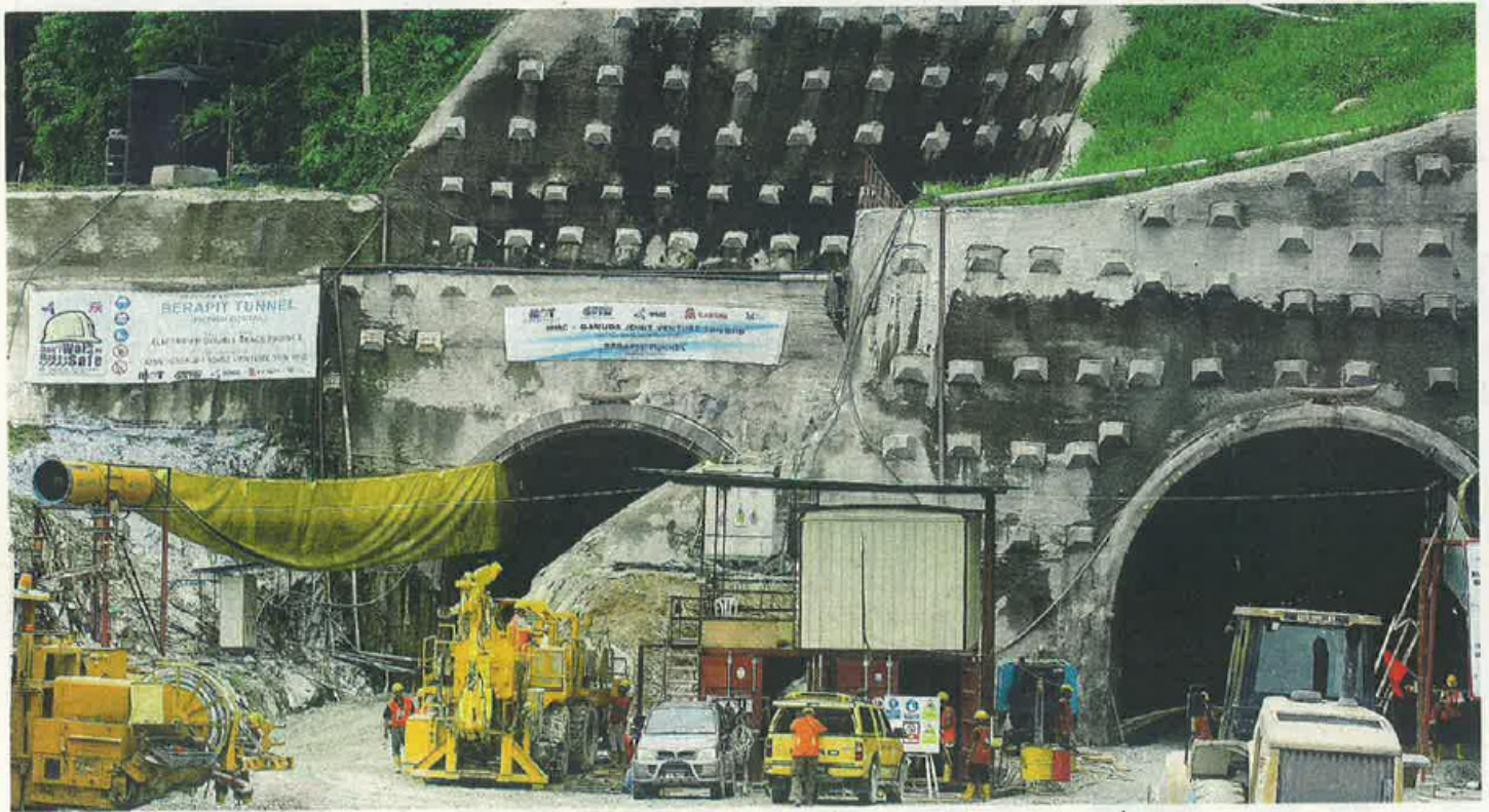
The Berapit twin tunnels in Padang Rengas have nine cross passages as part of their safety and maintenance feature. — NST picture by Ikhwan Munir
